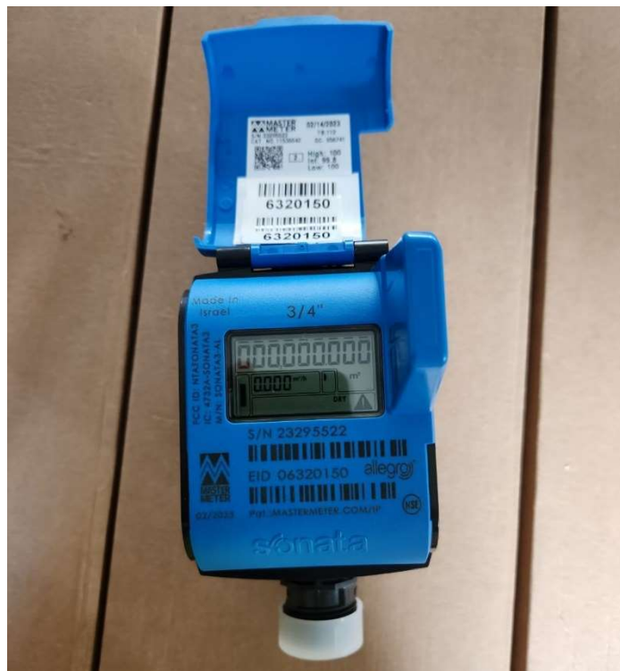
IMAGE | NEW METER, INSTALED UNDER THE AMI REPLACEMENT PROGRAM.
