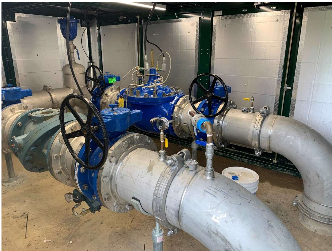
IMAGE | WATER INFRASTRUCTURE AT THE RESERVOIR SITE.
