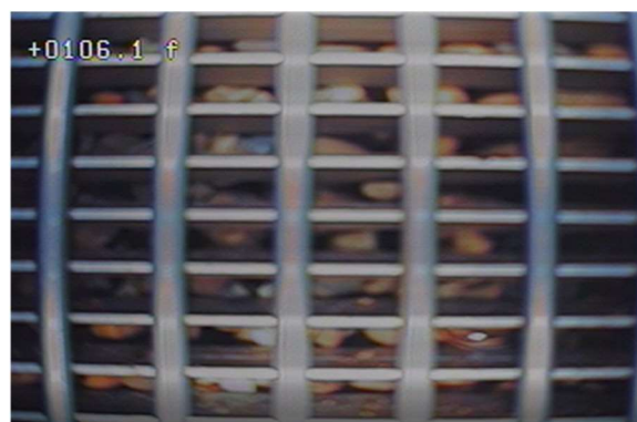
After chemical treatment ( most scaling has been removed )
